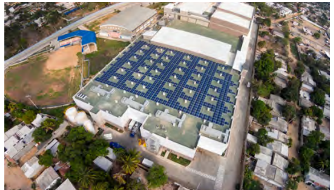
We have more than 16,520 solar panels in our shopping centers and warehouses; 5% more than in 2023 thanks to the launch of the photovoltaic plant in VIVA Wajira, Riohacha, Guajira.
